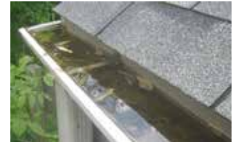
Clogged Gutters can be easily detected by spraying water onto the roof and watching for steady downspout flow.
